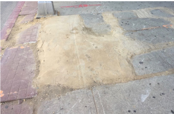
Inadequate sidewalk repair in the Heights
